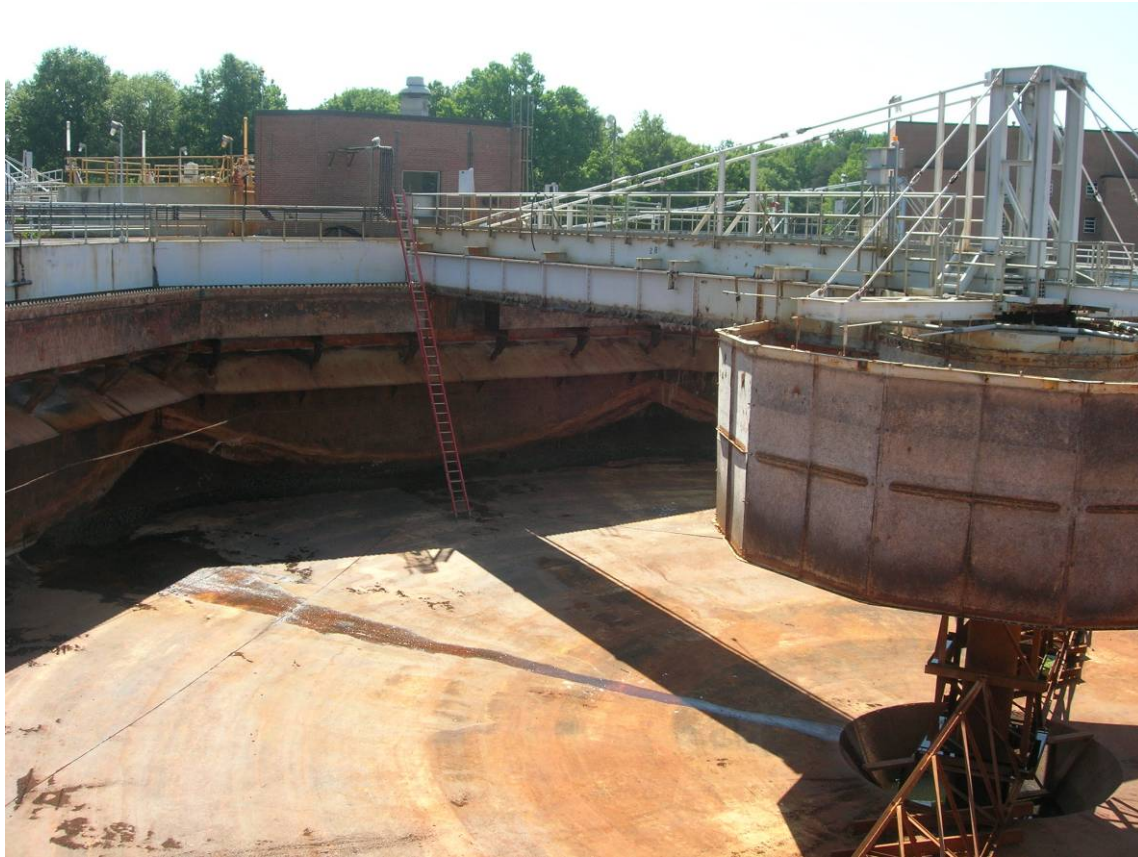
Empty tertiary clarifier at Noman Cole PCP
